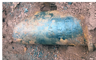
Warren Foundry gray iron pipe circa 1886 recently unearthed has a relatively smooth surface and raised lettering from pit casting.
